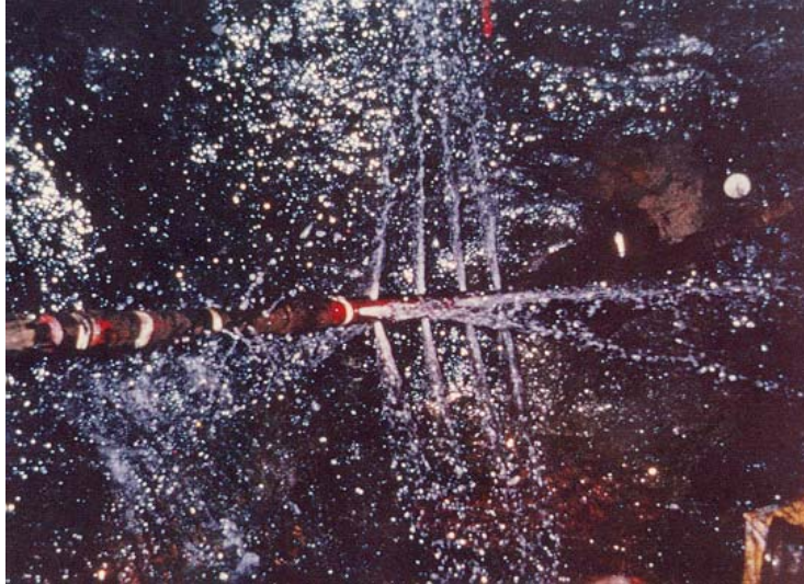
Figure 9. Straddle packer used by REI Drilling, Inc. to hydraulically fracture directionally drilled boreholes at the Soldier Canyon Mine.
